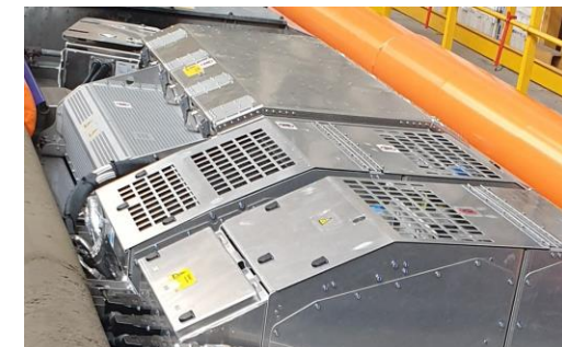
Batteries on roof of EMU
